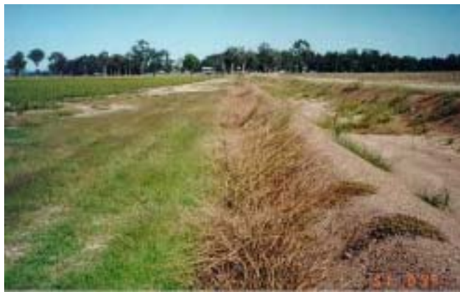
A channel bank in northern NSW a day after it was flamed
