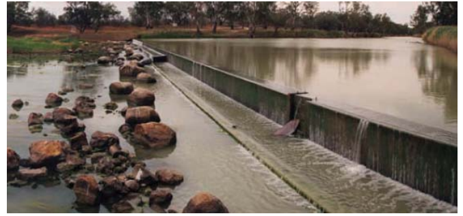
The Brewarrina weir. The existing fishway is inadequate and work is now underway to improve passage for native fish. Photo: David Cordina
