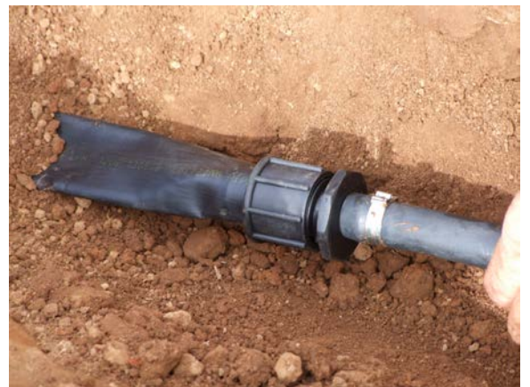
Connection to the drip tape. Image: S. Priest
