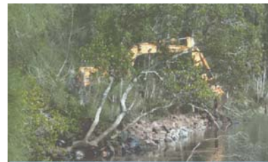
An excavator with a long arm grab was used to construct the rock fillets. Photo: D.Kirkness
