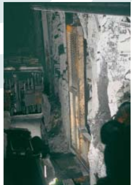
The ABM 20 rib support protection system in place against the rib
