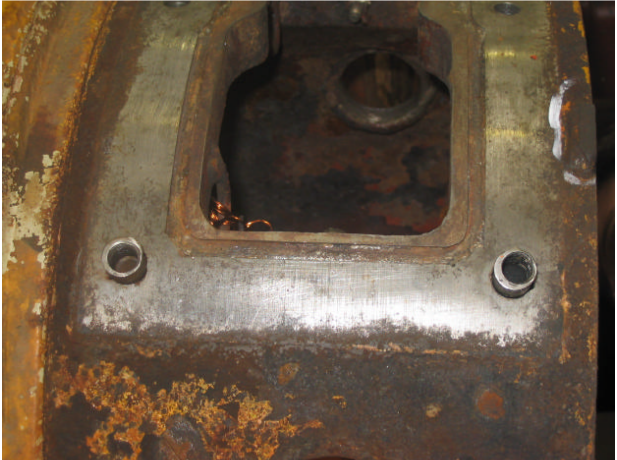
Figure 2. General view of side cover of Motor A showing partially removed inserts.
