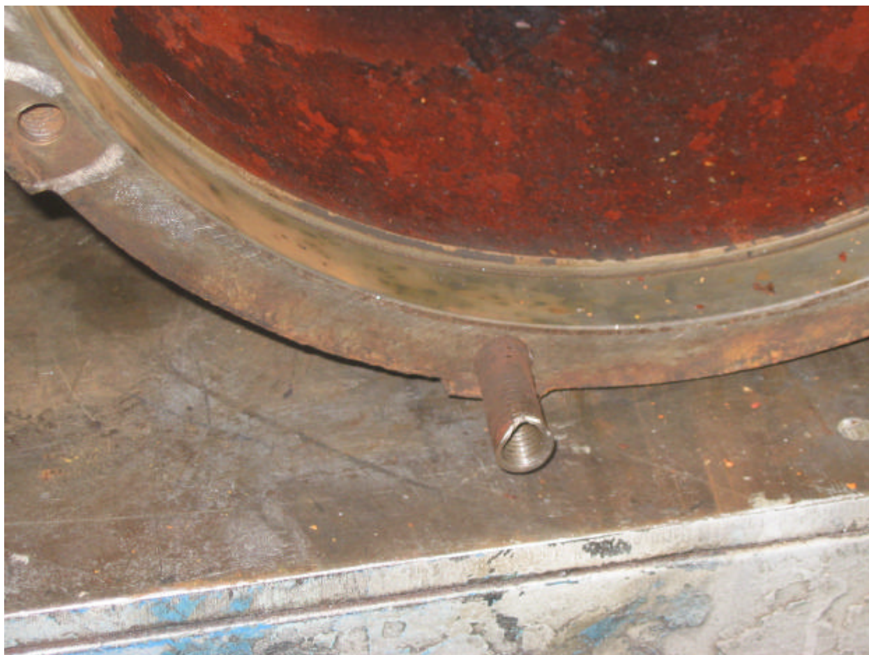
Figure 3. Detail of the partially extracted insert from Motor A.
