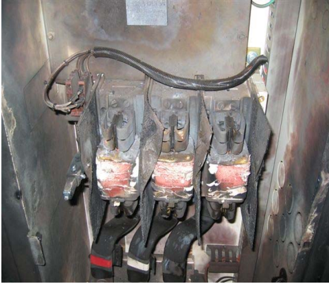
Failure 1: 630 amp 690v fuses Cat. Bussman Czech 630 NH3G-690
