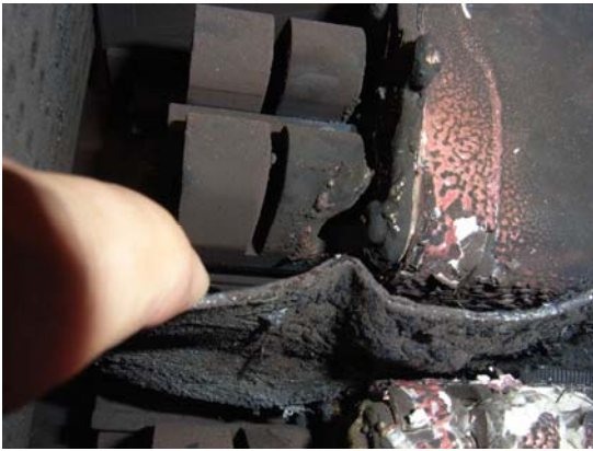
Failure 3: 500 amp 690v fuses Cat. Bussman OEZ Czeck 500 NH3G-690
