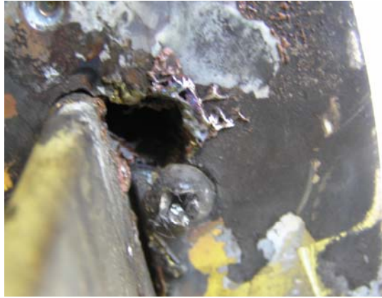
Failure 2: 630 amp 690v fuses Cat. Bussman Czech 630 NH3G-690
