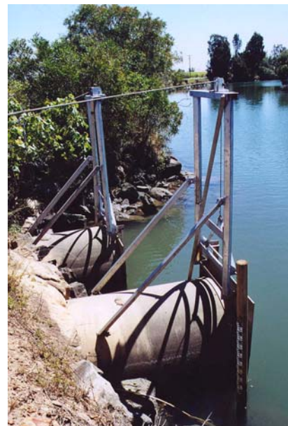
Floodgates are being modified with the help of funding from the Northern Rivers CMA.
