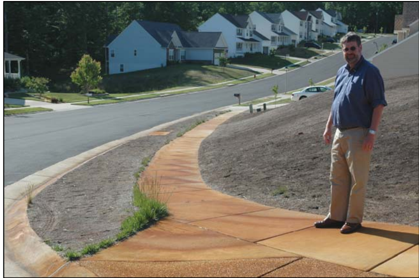
Iron (hydr)oxide coatings on sidewalk.
