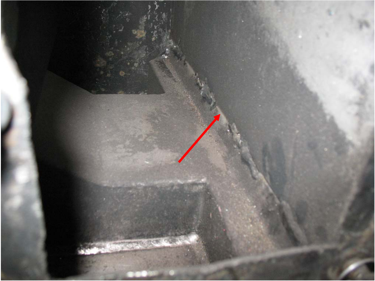
Photo – Showing weld discontinuities.
