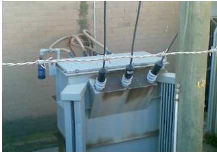
Transformer out feed cabling overheating
