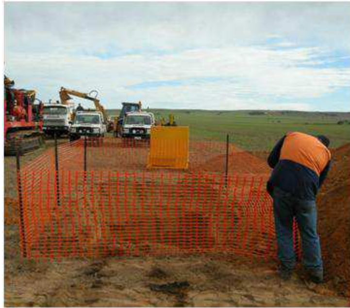
Photo 4: Typical barricading of sump during use
