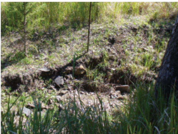
The toe of the old slip starting to erode
