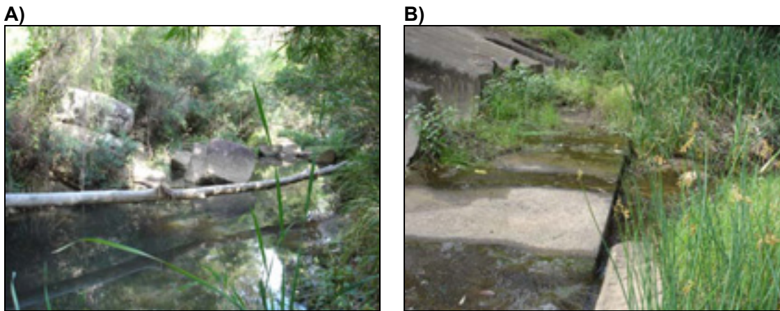
Figure 3. Wedderburn Weir, Georges River (27/01/2005) showing A) habitat downstream of structure, B) apron with 200mm headloss and minimal flow depth (downstream side).
