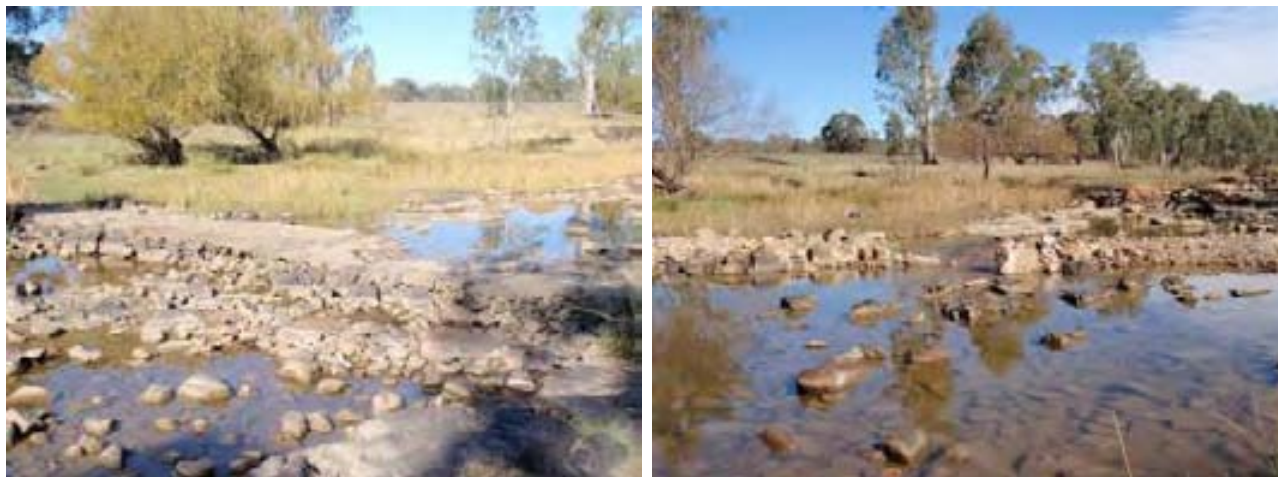
Little River causeway before and after remediation. Photos: Kirby Byrne NSW DPI
