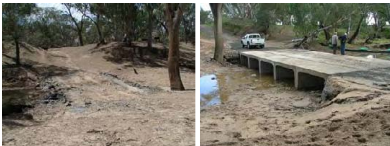
Above: This 'fish-unfriendly' pipe culvert has been replaced by a palatial new box culvert crossing. Photos: Nathan Reynoldson NSW DPI
