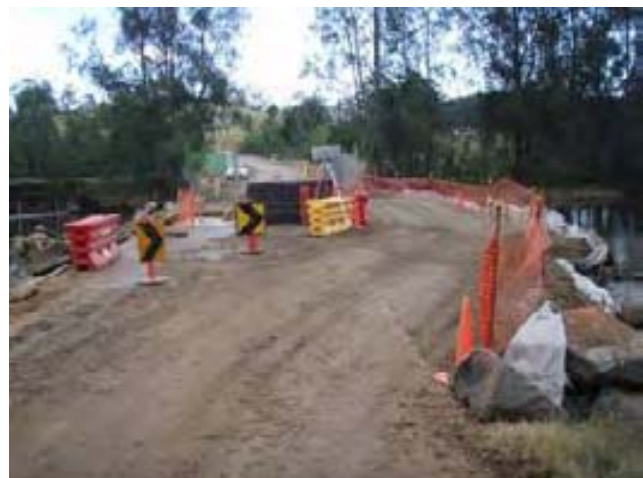
Above: Traffic diversion around the culvert works. Photo: Ian Macgrath, Eurobodalla Council
