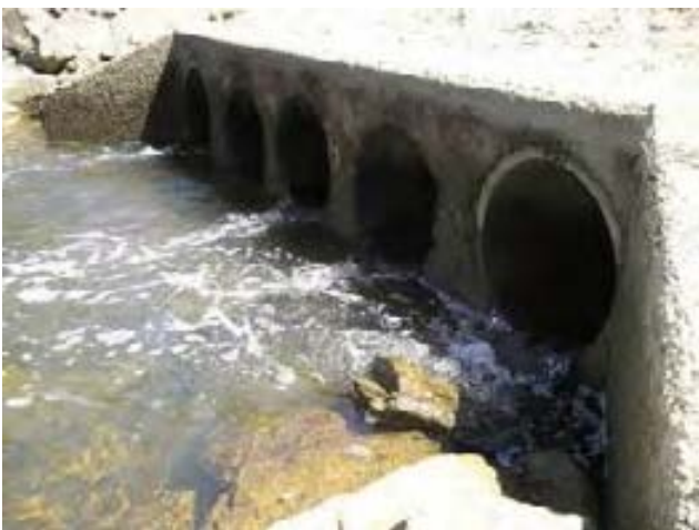
Above: The problematic causeway pipes at low tide. Photo: Scott Nichols NSW DPI
