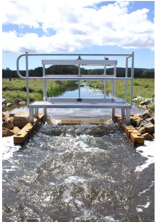
An “Overshot and Undershot” gate, a similar structure to that installed at Imesons Swamp
