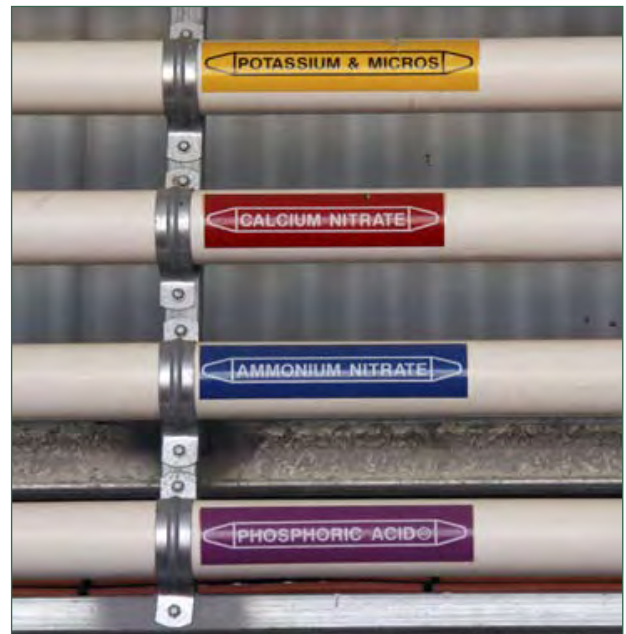
Figure 3. PVC pipes taking separate dissolved fertilisers to the injection point.
