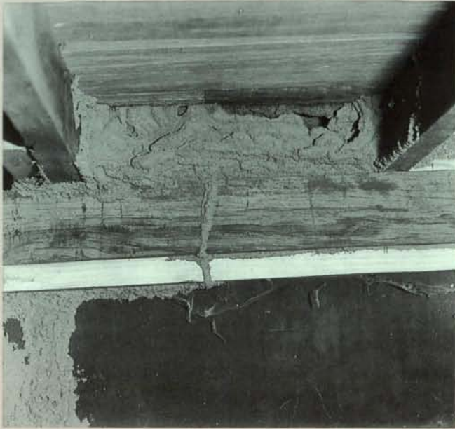
Mud plastering and galleries built by subterranean termites in obtaining access to a suspended floor
