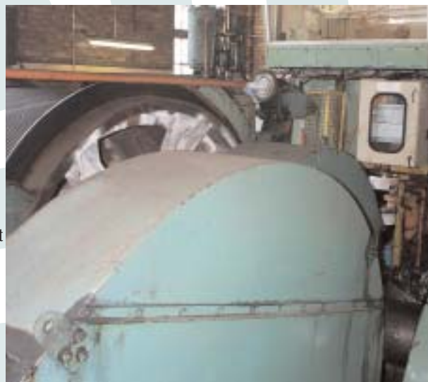
Mine management should ensure that risk assessments are carried out to identify all hazards arising from all winding activities.
