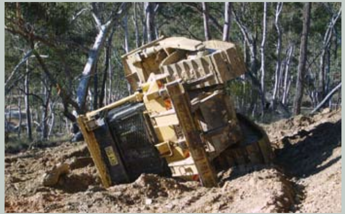
Wearing a seatbelt helped protect a bulldozer driver from suffering serious injury or death when the vehicle rolled over while working on a slope. Fitting appropriate passenger restraints and protective devices should be considered for plant used at mines.
