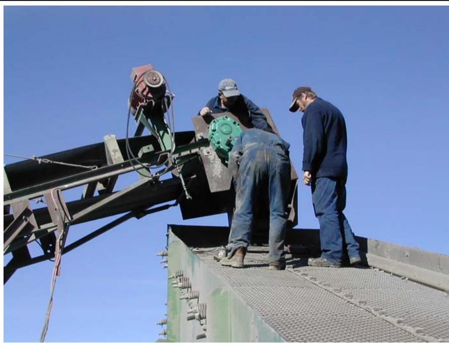
Plate 8.1: Unsafe work procedures whilst repairing conveyor head pulley drive
