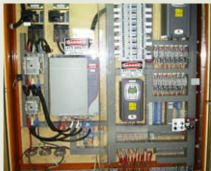
An improved electrical installation. The standard of installations viewed during the program varied greatly.
