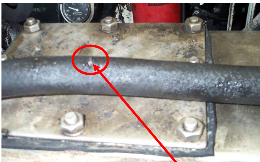
Pin Hole in the hydraulic hose
