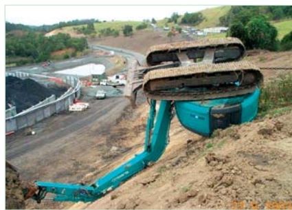
Small excavator roll over
