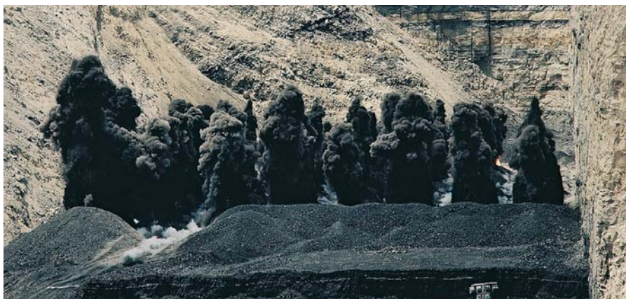
Using explosives has potential for injury
