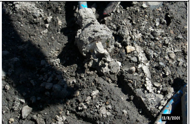
Plug not suitable for the environment, poorly installed and poorly maintained
