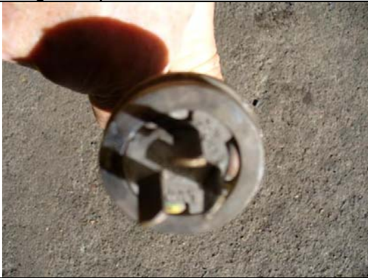
Plug inadequately IP-rated
