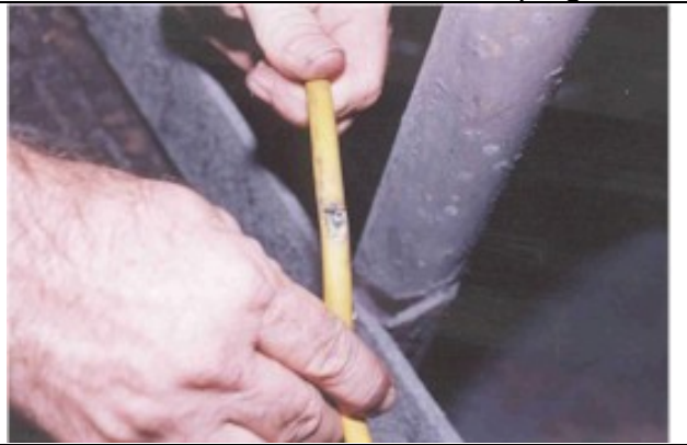
Damaged extension lead due to poor installation practices.
