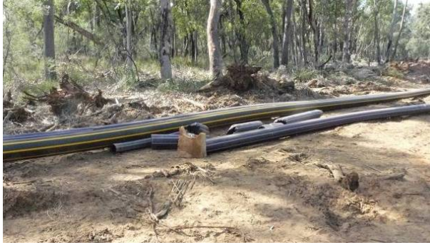
Showing broken pieces of pipe found near the pit from which the pipeline was being recovered.
