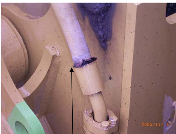
Corroded hose end
