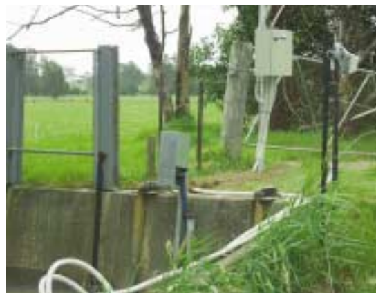
Smart gate installation.
