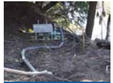
The electric pump unit which replaced the diesel pump. It is skid mounted to allow it to be hauled above flood level.
