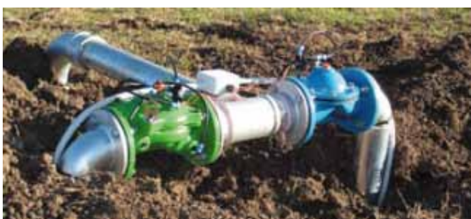
Electric control valves on mainline and laterals.
