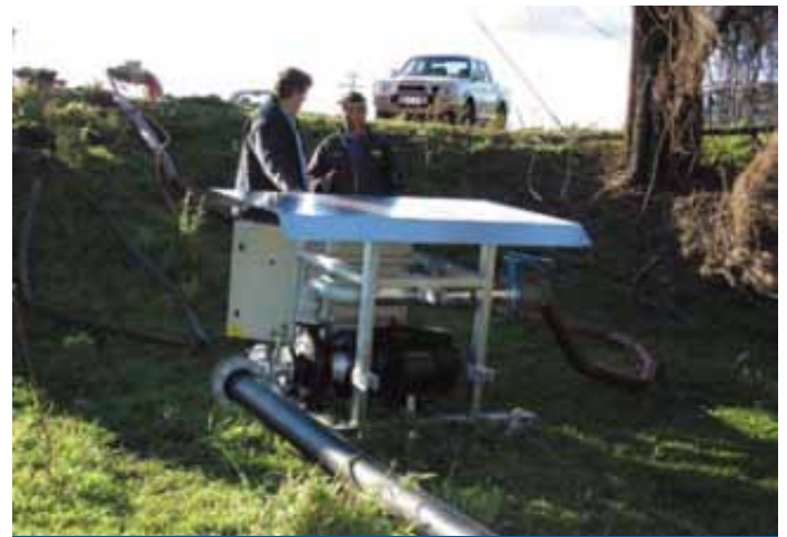
Movable pump installation on river bank.
