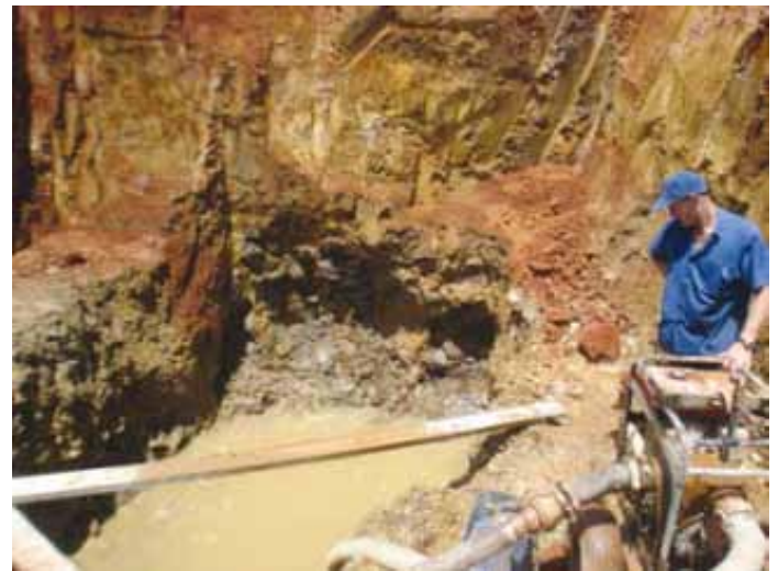
Ben Hurrell pumping down water from the spring under the dam wall.
