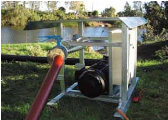
Skid mounted electric pump unit which can be moved out of flood zone.
