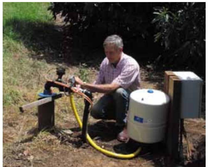
The small bore with submersible pump and pressure system.
