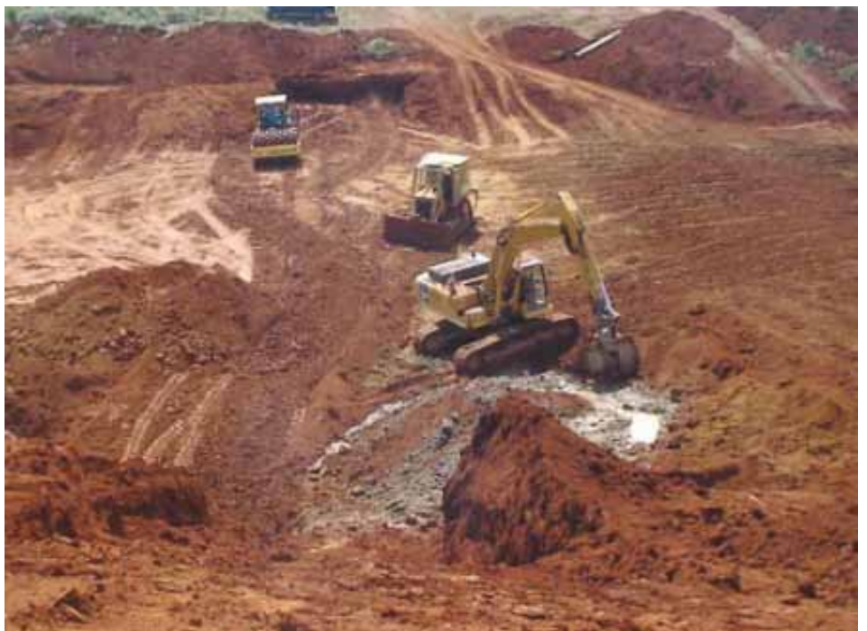
The excavator is working on sealing the spring while the bulldozer and roller compact the dam wall. This will ensure a secure dam.
