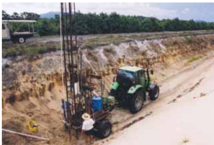
Drilling and installing groundwater system into the sandy soil profile under the orchard. Roots only extend into the very shallow top grey layer which severely limits water available to the crop.
