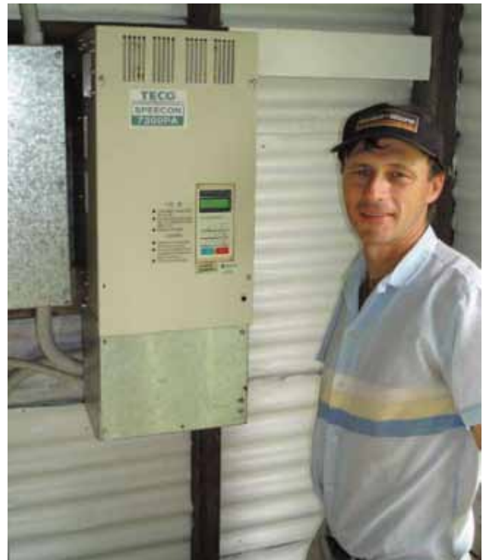
Andrew Harwood stands by the control panel for his irrigation pump. The pump draws from a storage developed in a depression.
