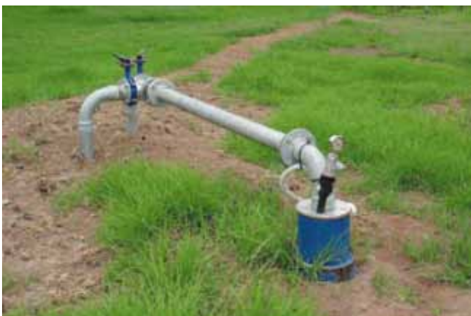
This small bore with submersible pump 'tops up' the storage since flow rates are too low to use directly in the irrigation pump.
