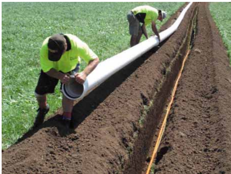
Installing the mainline and the controls and power line to the central pylon.
