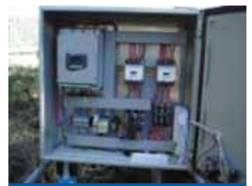
The control unit for the electric pump.
