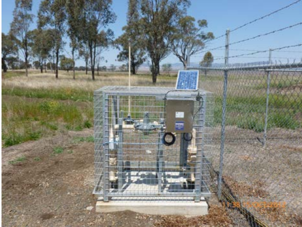
Figure 2: The remote monitored gas meter at 'The Point'.
