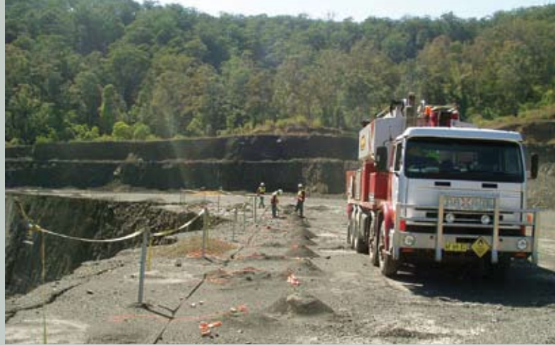
Specially fabricated lightweight posts form a barrier near the bench face at Kulnura Quarry, reducing the risk of a fall.
