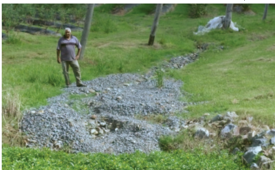
Subsurface drainage improves the central flow line
