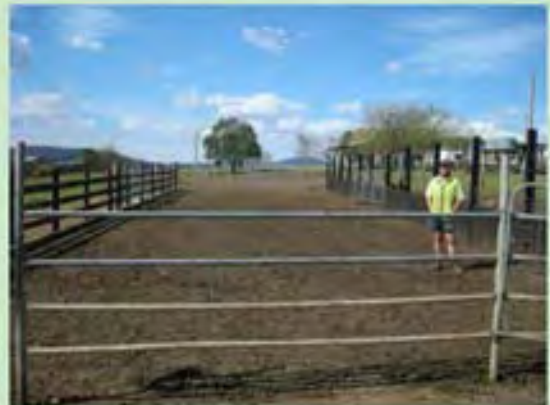
Below: The trafficable solids trap has been constructed using a mould developed by the Mid-north Coast Dairy Pasture Council and funded by Subtropical Dairy.
