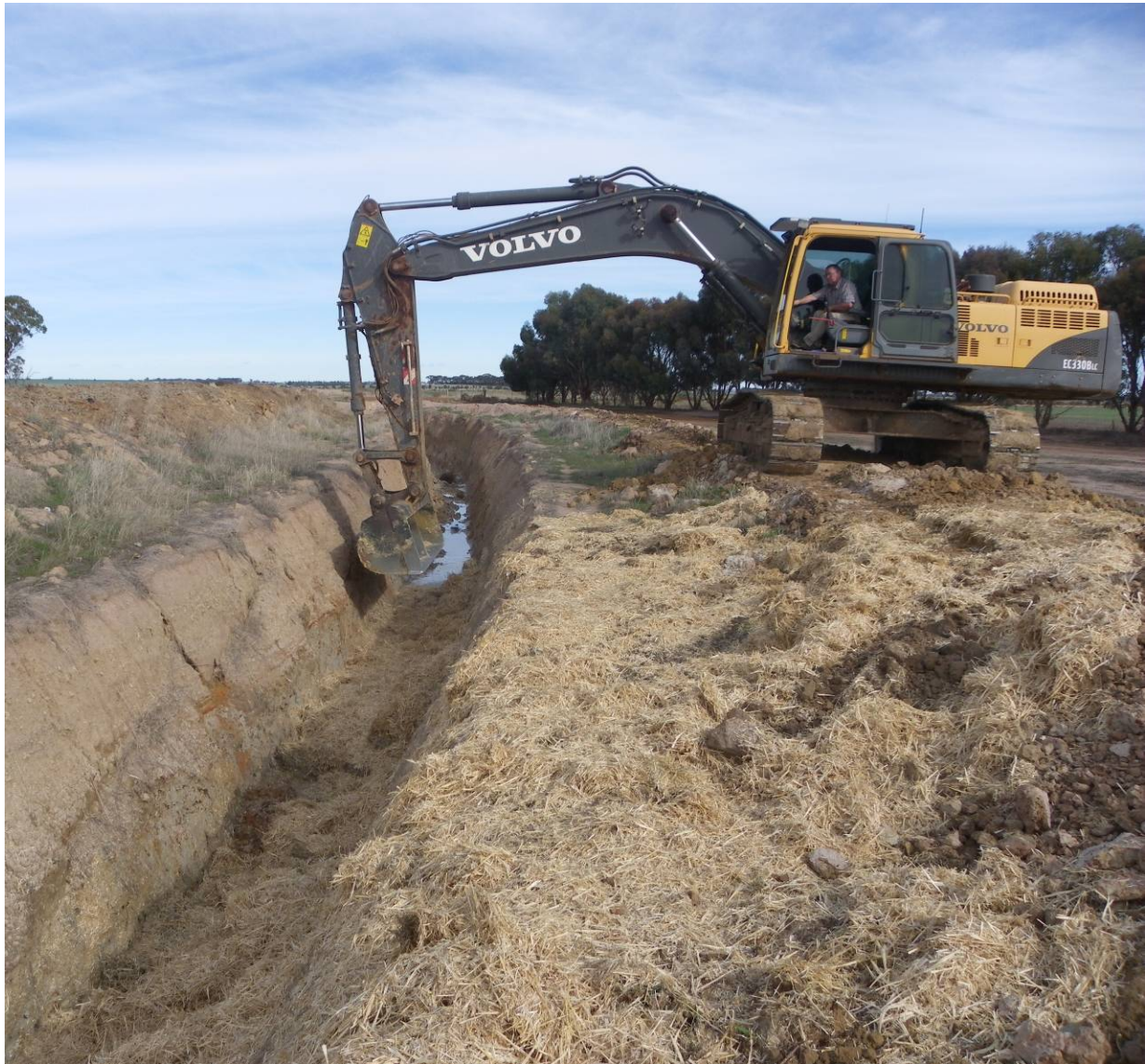
Compacting straw to form a simple in-drain anaerobic treatment system for acidic saline discharge treatment
