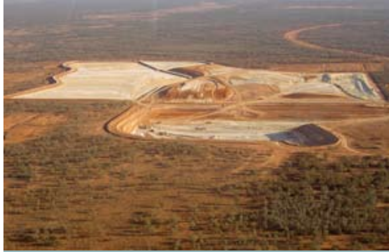
Ginkgo mineral sands project in the Murray Basin. The mine will commence production in late 2005.
