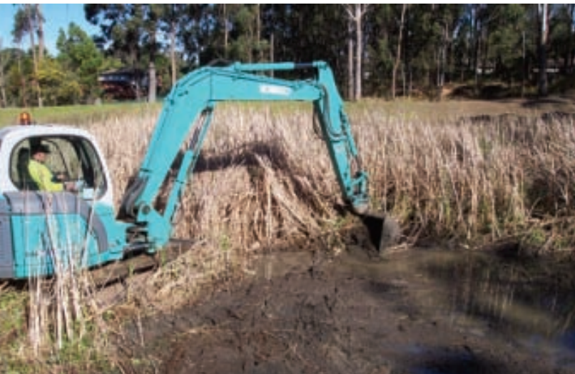
A 10 m × 10 m area was excavated to a depth of 150 mm. Photo: Graham Prichard
