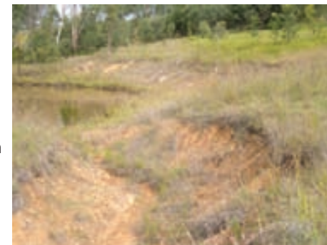
An eroding dam spillway
