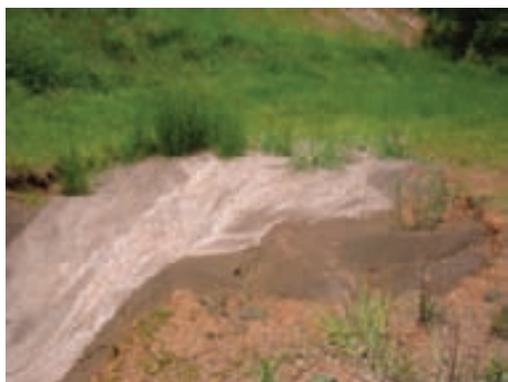
A sediment fan means erosion upslope.
