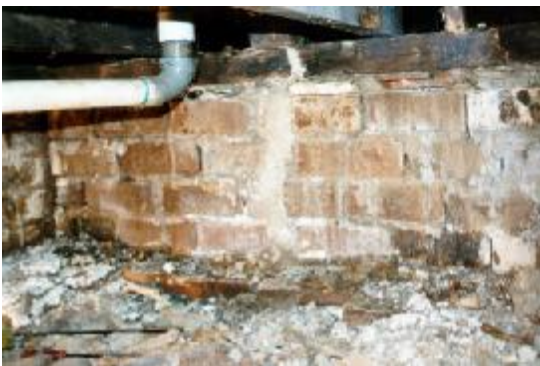
Figure 2. Main gallery by which termites enter a building. A nearby leaking water pipe probably encouraged termites into this part of the building.
