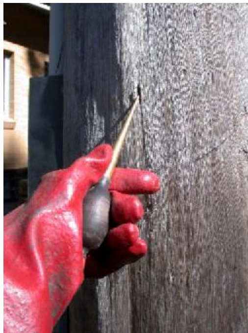
Figure 4. Termite dusting an infested power pole.
