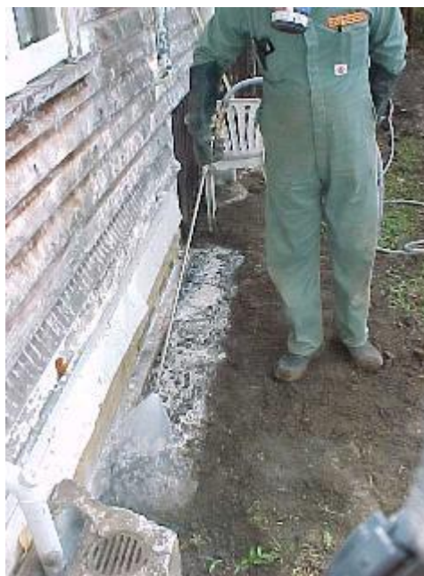
Figure 5. Termiticide application to a building perimeter by trenching and treating the backfill.
