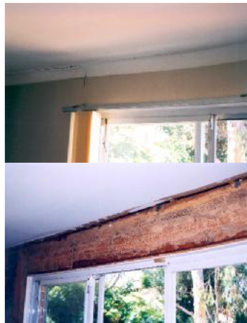
Figure 3. Sagging cornices and warping plasterboard (top) can be indicative of termite activity underneath (bottom).
