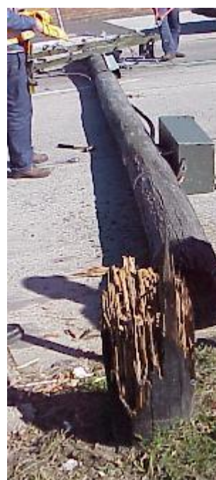
Figure 1. Power pole failure resulting from termite attack.
