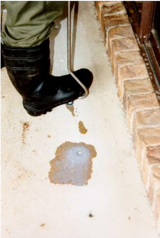
Figure 6. Injecting termiticide through holes drilled in a slab. Holes are sealed after treatment.
