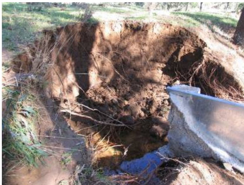
Figure 18 Bank erosion during flood event June 2007.
