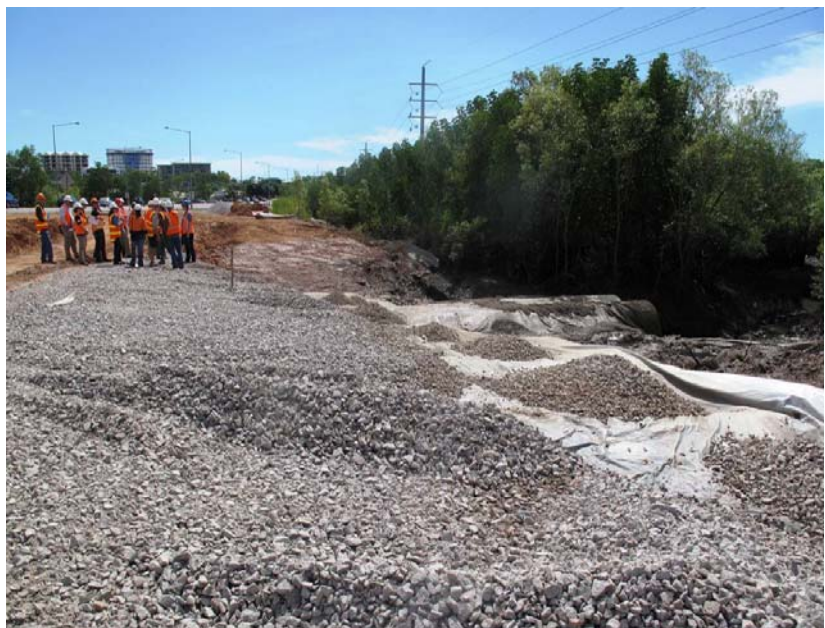
Tiger Brennan Drive being widened over disturbed areas of acid sulfate soils
