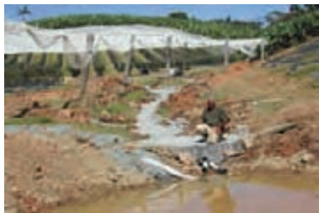
This subsurface drain manages low flows to allow vehicle traffic through.
