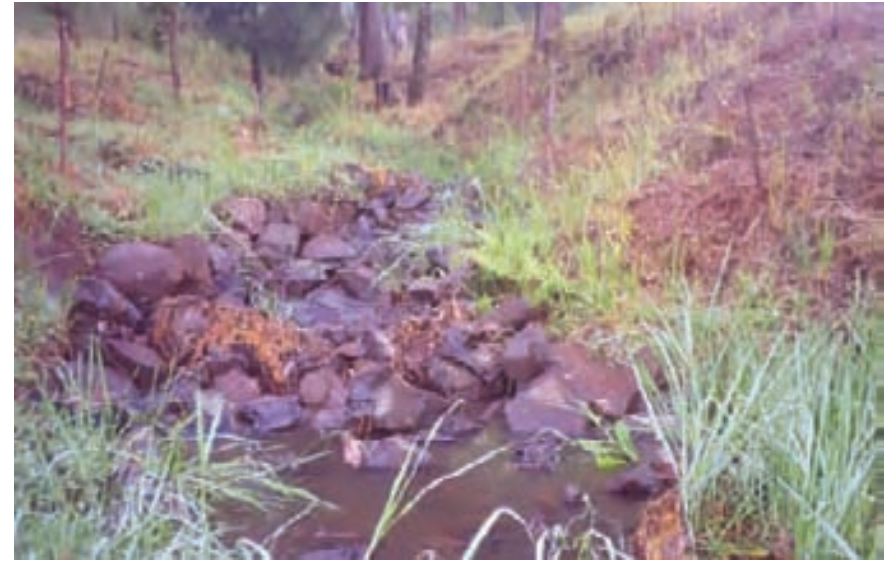
Protect persistently scouring channels with rock.
