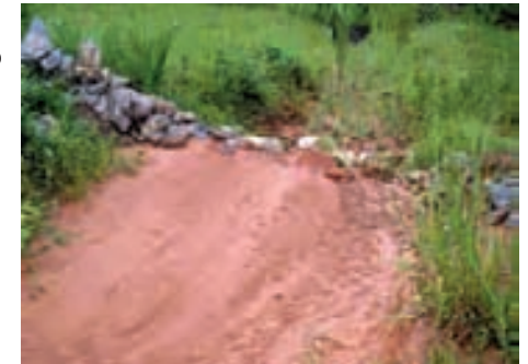
Sediment needs to be removed to maintain the effectiveness of this structure. Source: Michael Frankcombe IECA
