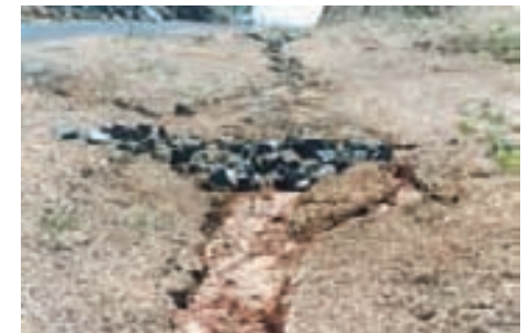
This rock check dam is failing because the rock does not extend far enough up the channel sides, and the lowest point is not in the centre.
