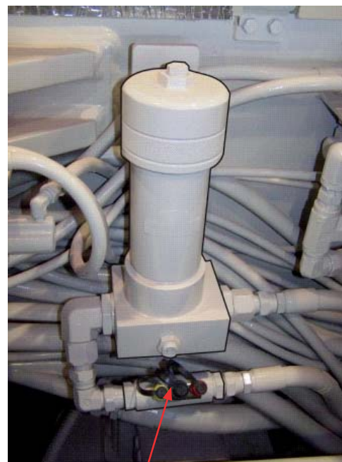
UCC Inline Sensor Test Point
