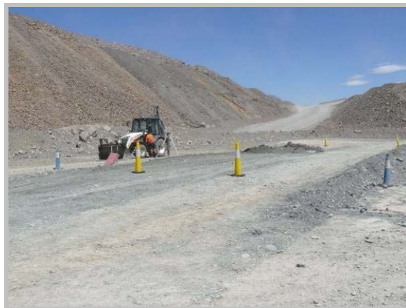
The photo shows yellow coloured cones placed around an operating backhoe at CVO site.
