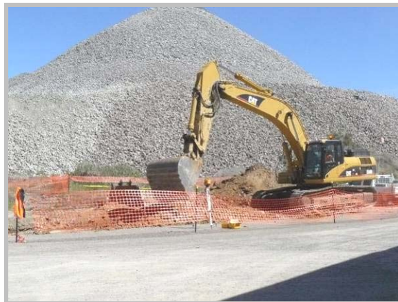
The photo shows a construction zone using mesh barrier tape erected around an operating excavator at CVO site.
