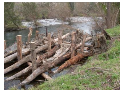
The log jam in the construction phase. Logs were sourced from nearby highway construction. Photo: Kylie Russell
