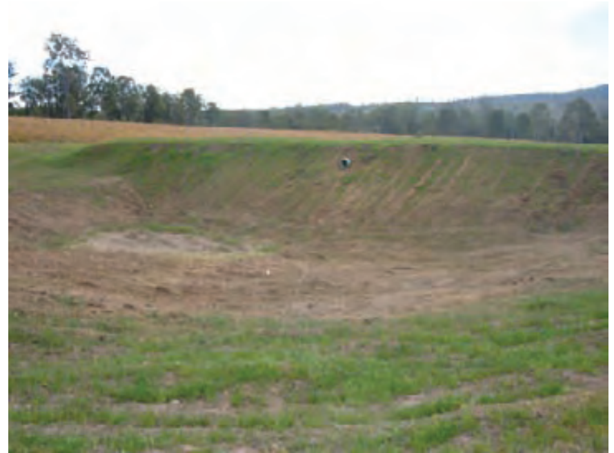
A newly constructed gully dam, showing the excavation, embankment, spillway and a trickle pipe for low flows.
