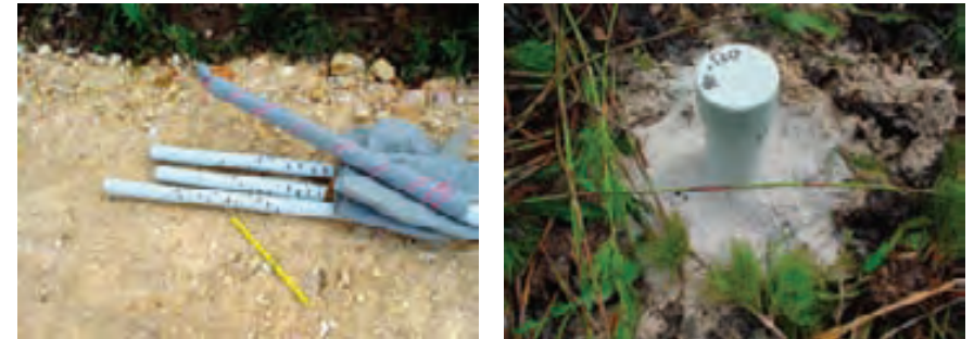
Slotted pipes for use as piezometers. In the ground only the top of the pipe is visible. Source: Keith Bolton
