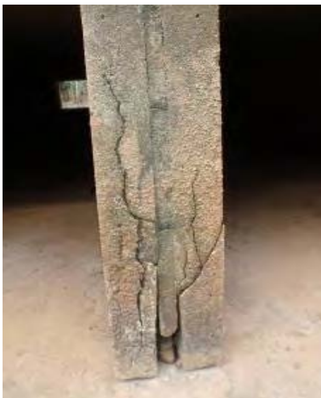
Acid-damaged pylon Photo: Jeremy Manders
