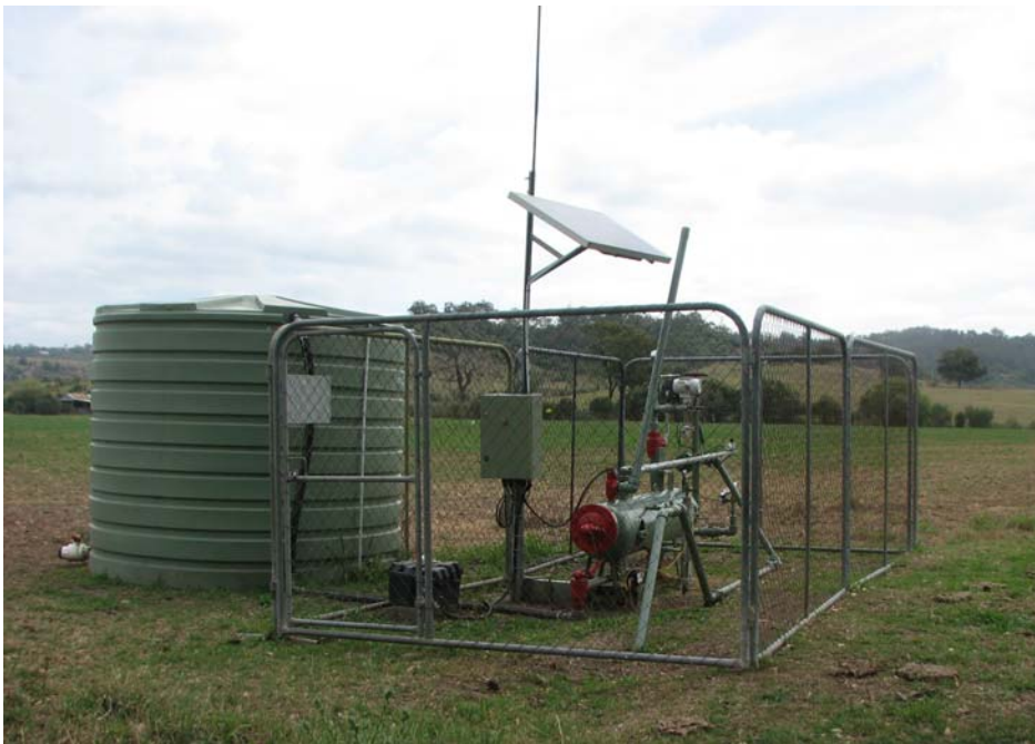
Figure 1: Coal seam gas well have been operating at Camden NSW since 1999
