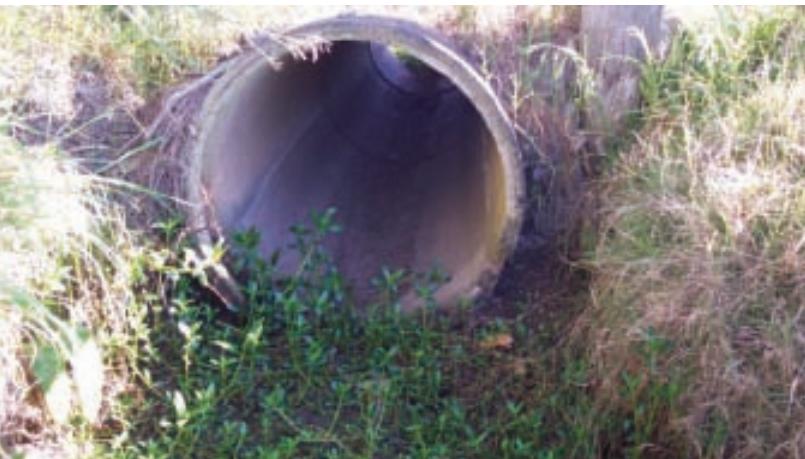
Infestation at culvert in need of containment. Photo: Graham Prichard
