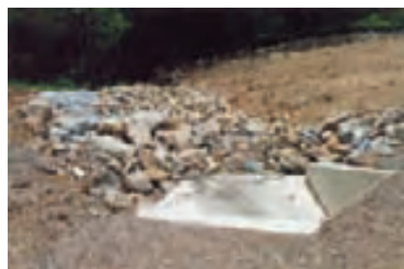
Rock protects the batter where this culvert emerges. Source: Tim Duckett IECA
