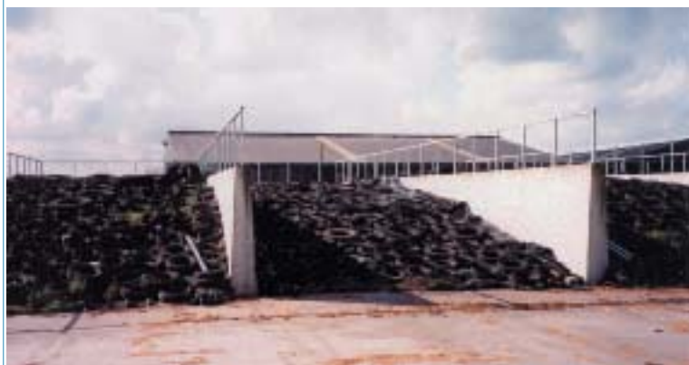
Guard rails are strongly recommended on the walls of above-ground bunkers and portable clamps to reduce the risk of tractors slipping over the edge of the wall when rolling silage. Photograph: R. Morris
